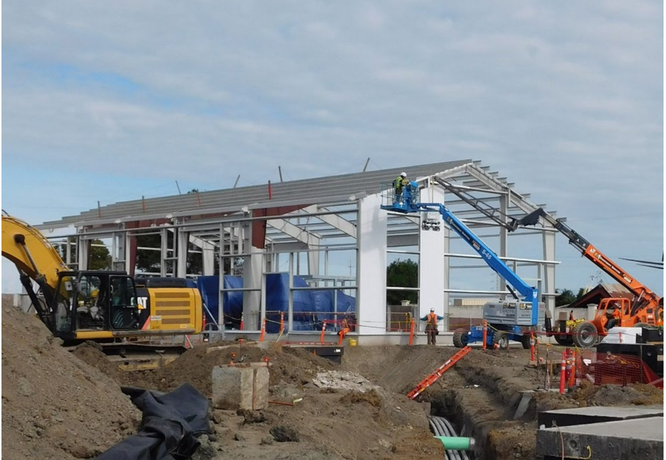
New Standby Power Building
