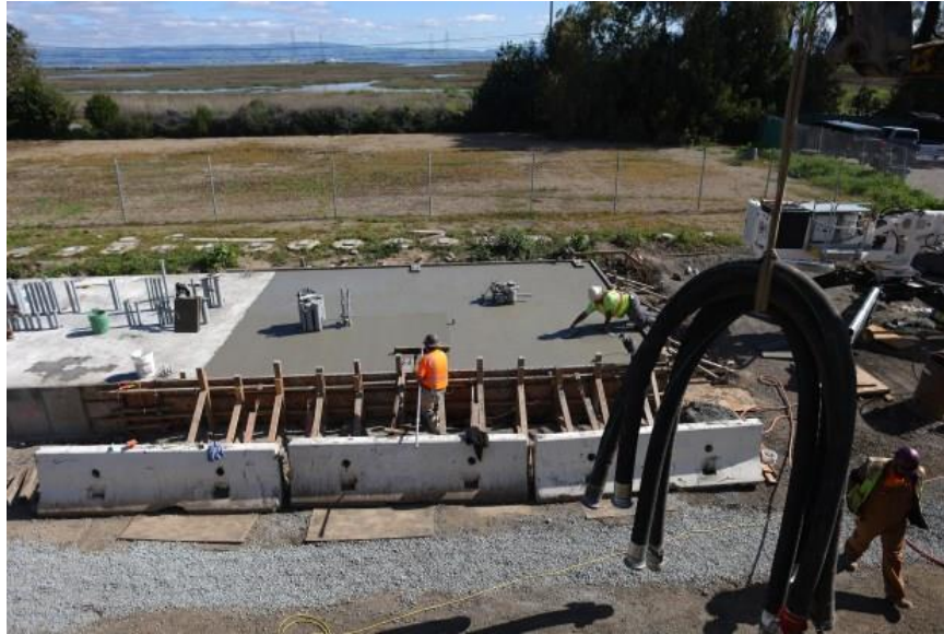
Construction crew members work on the foundation of a new power distribution building at the Regional Water Quality Control Plant on Thursday, March 21, 2024, in Palo Alto, Calif. The plant is undergoing a $369 million upgrade project. (Aric Crabb/Bay Area News Group)
