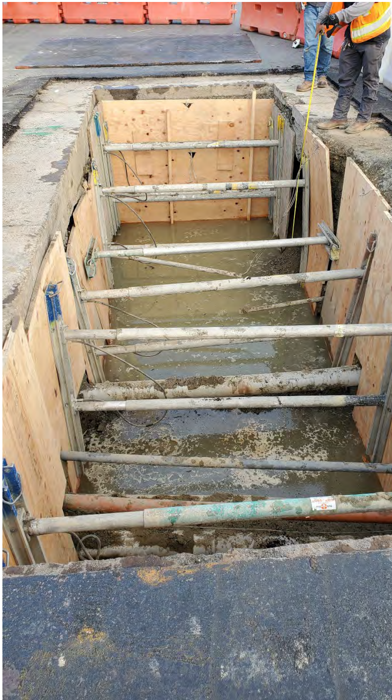
Figure 4 – Groundwater Encountered in Excavation of Westernmost Section
