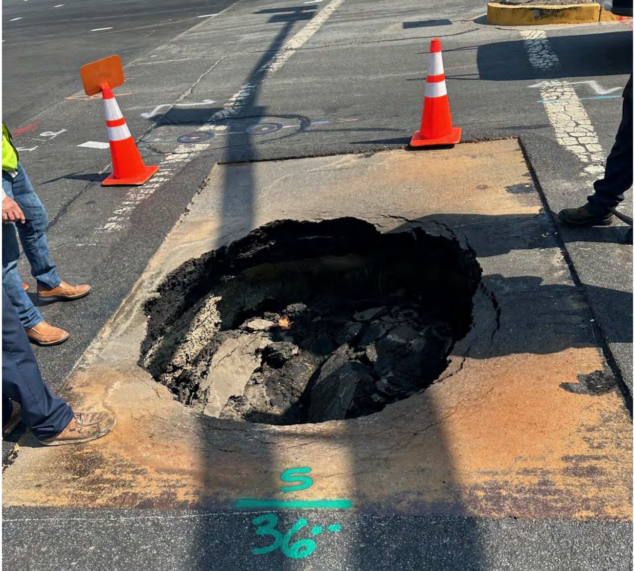
Figure 2 – Sinkhole at Intersection of Cushing Parkway and Auto Mall Parkway
