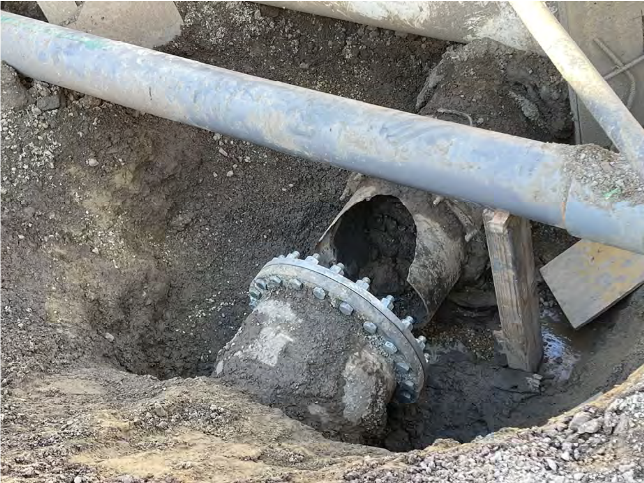
Figure 3: Existing Pressurized On-site Drainage Pipeline Failure
