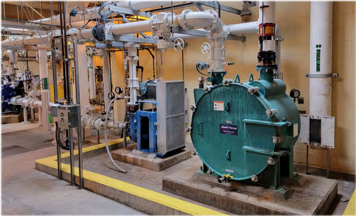
Figure 7 – Sludge Heat Exchanger
