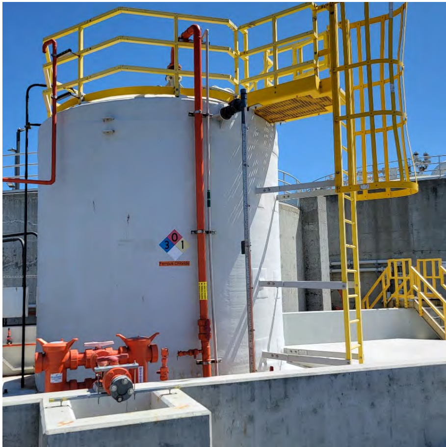
Figure 12 – Iron Salts Chemical Tank
