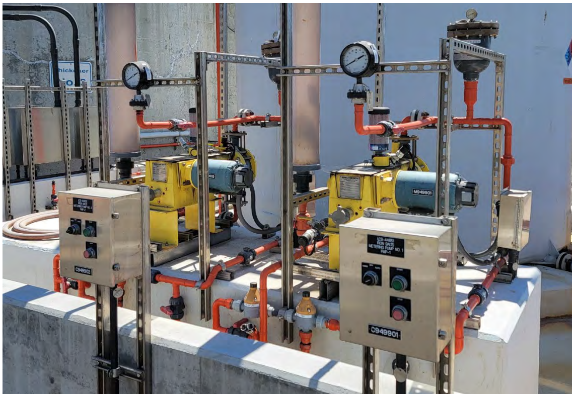
Figure 13 – Iron Salts Metering Pumps
