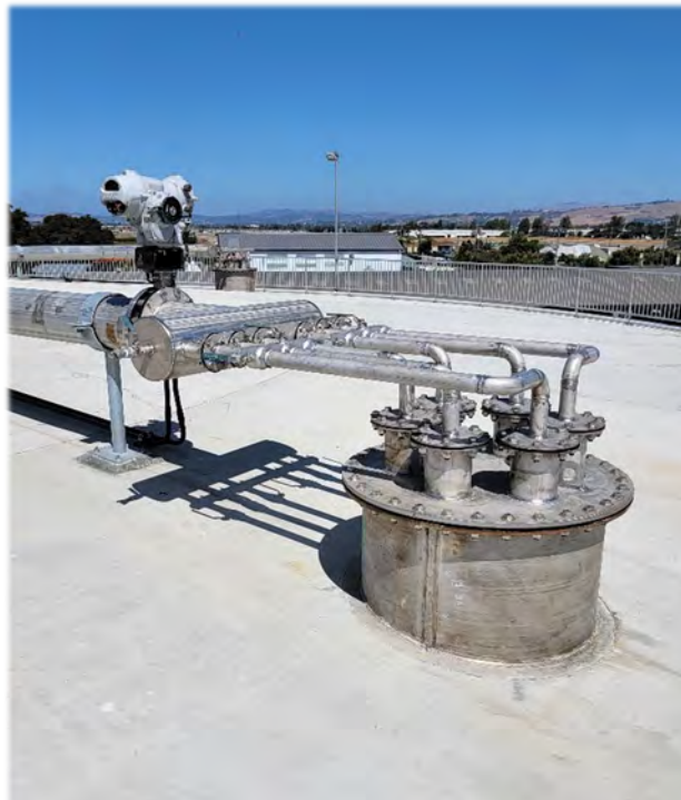
Figure 5 – Gas Lance Mixing Control Valve
