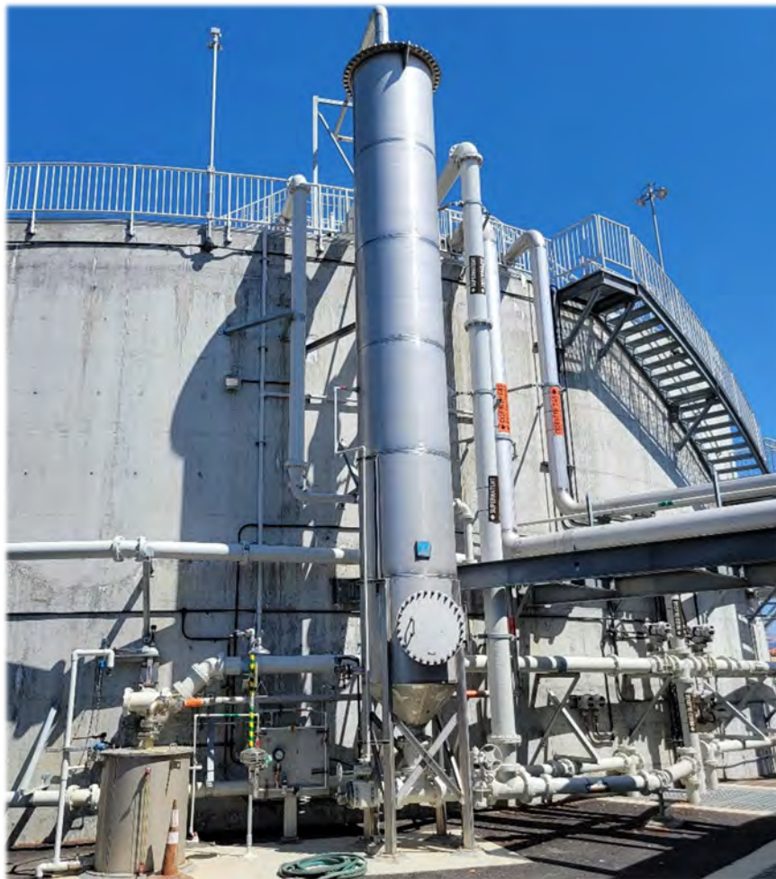
Figure 10 – Sludge Transfer Tank
