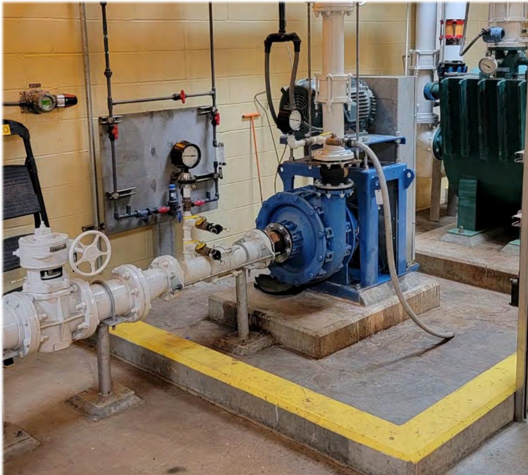
Figure 8 – Sludge Recirculation Pump
