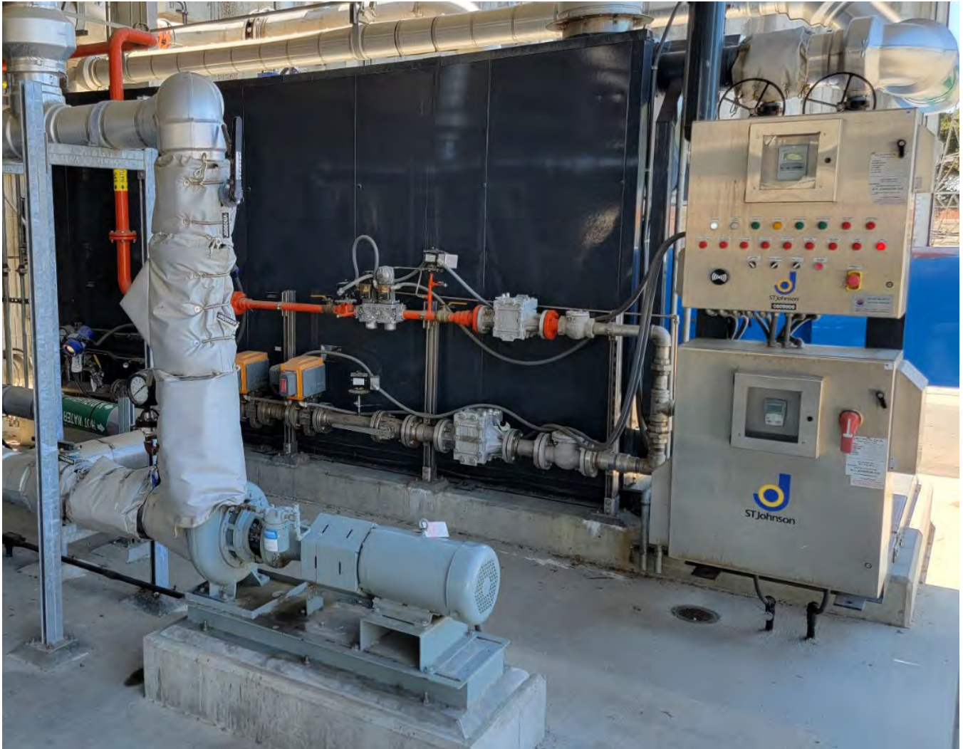
Figure 11 – Packaged Hot Water Boiler and Recirculation Pumps
