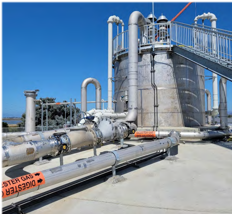
Figure 3 – Primary Digester No. 7 Stainless Steel Gas Dome
