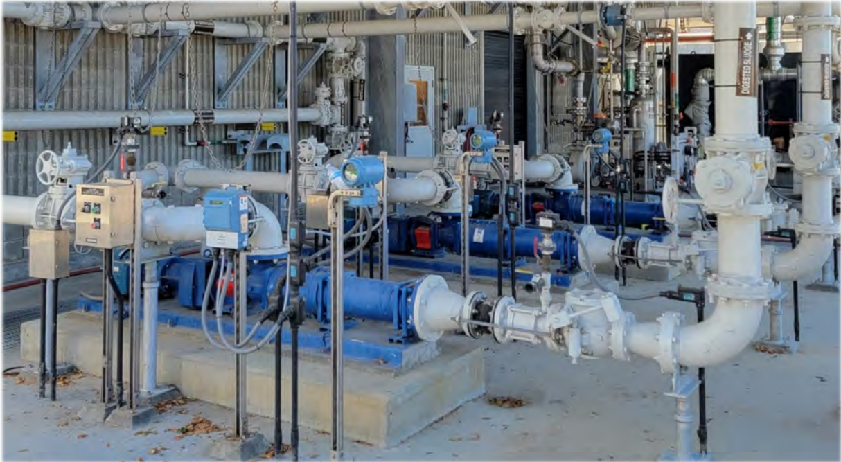
Figure 9 – Sludge Transfer Pumps
