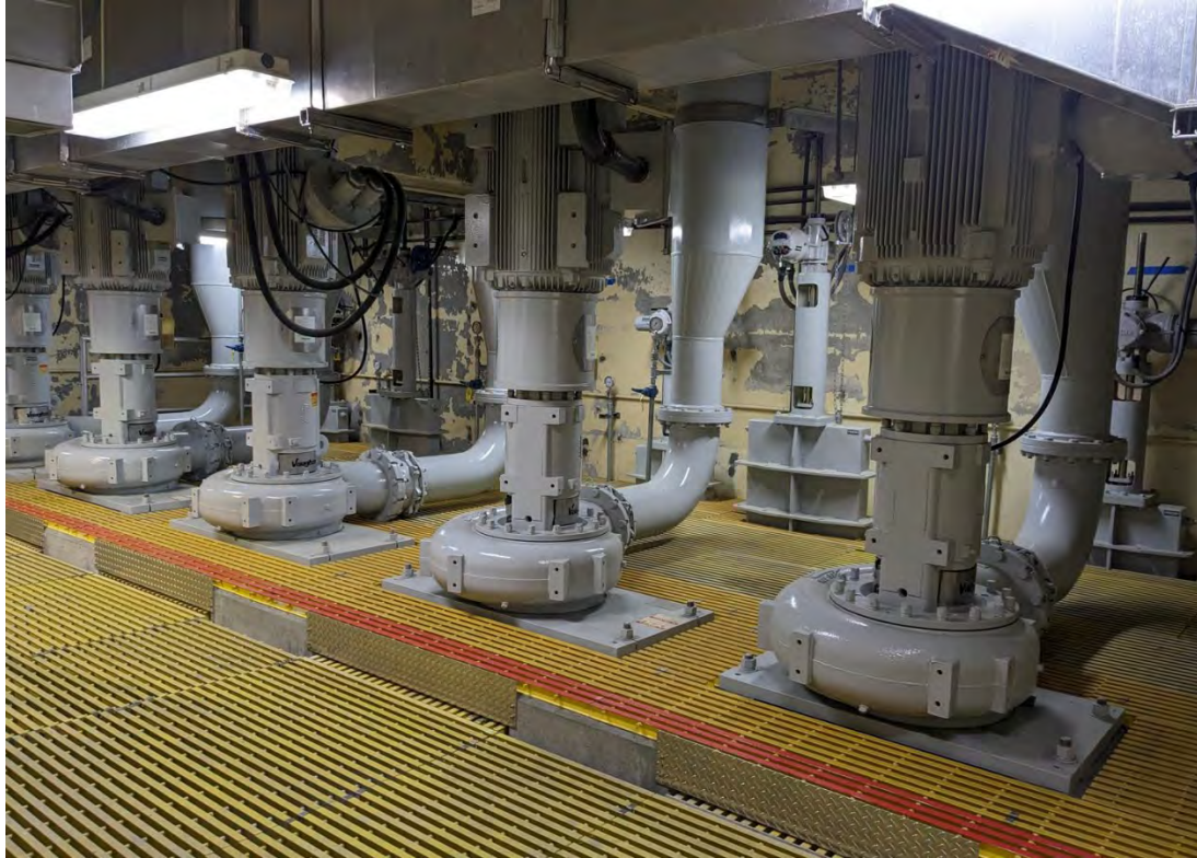
Figure 3 – New Wastewater Pumps and Piping at the Dry Well Basement
