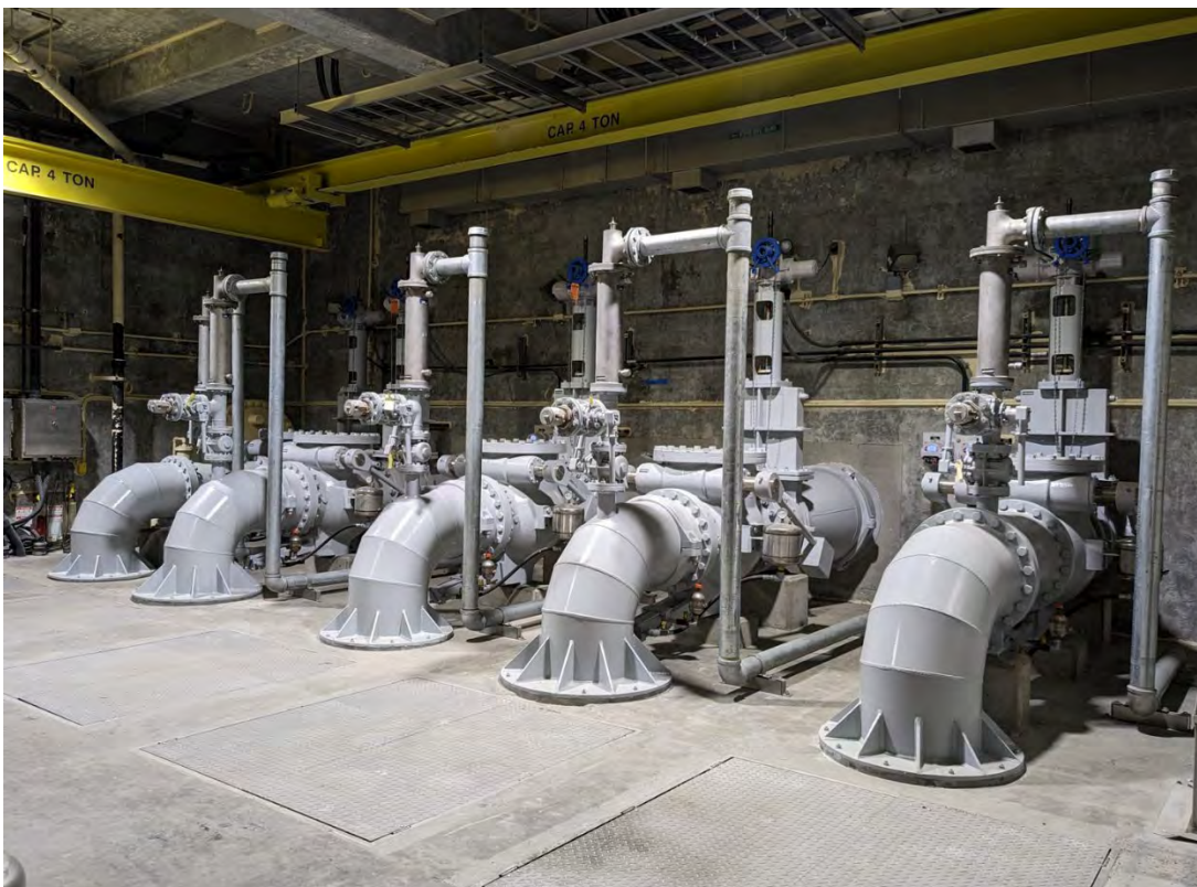
Figure 5 – New Piping and Valves at the Dry Well Intermediate Level
