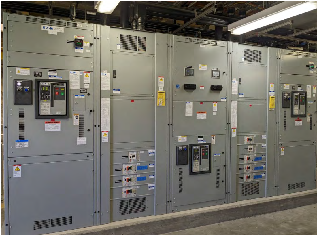
Figure 15 – New Electrical Switchboard No. 5
