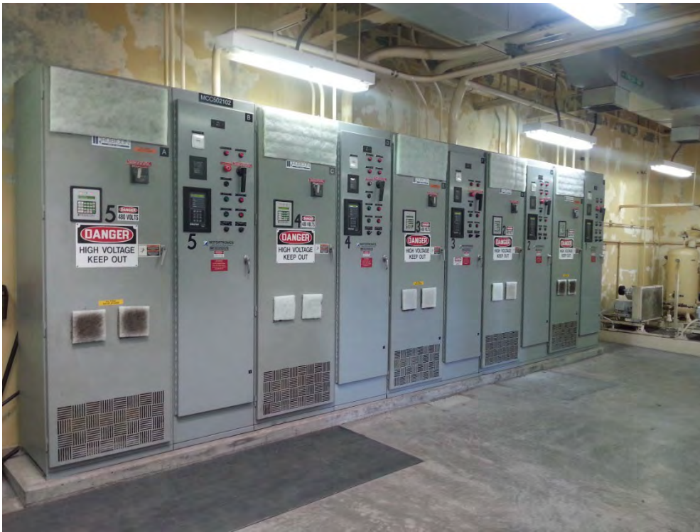
Figure 12 – Old Variable Frequency Drives for Wastewater Pumps
