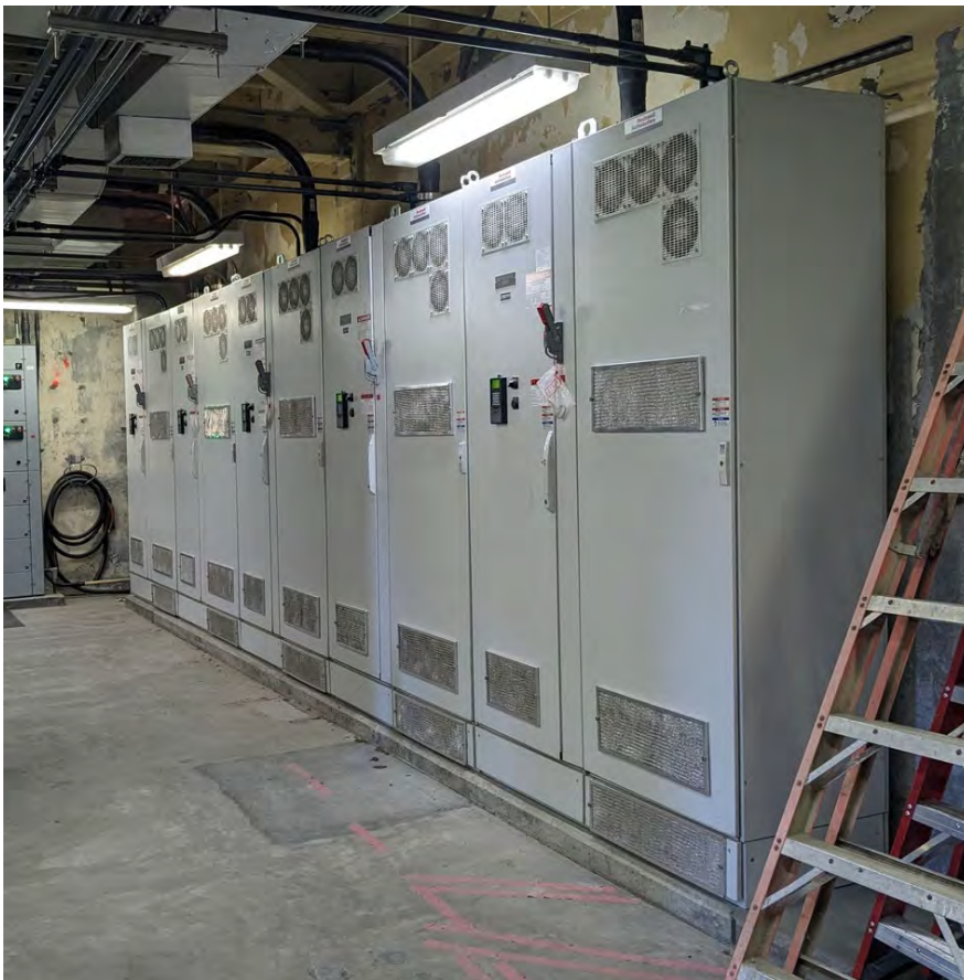
Figure 13 – New Variable Frequency Drives for Wastewater Pumps
