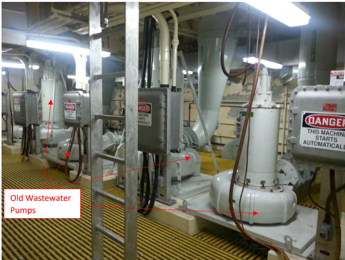
Figure 2 – Old Wastewater Pumps and Piping at the Dry Well Basement
