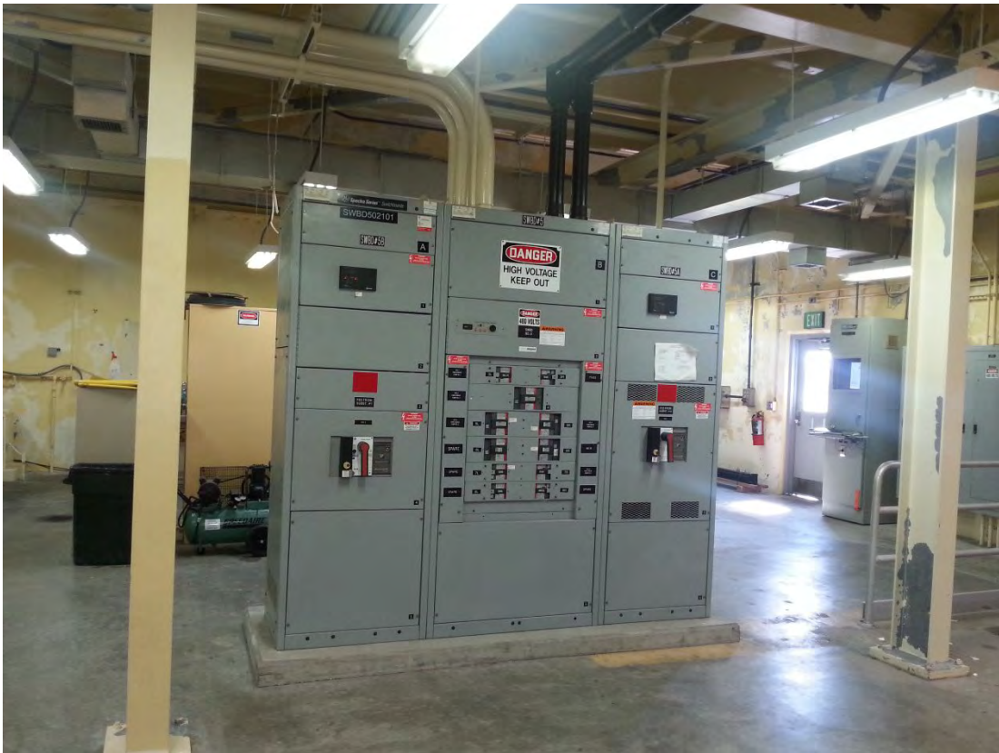
Figure 14 – Old Electrical Switchboard No. 5
