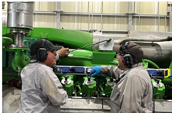
Mechanics working on the cogeneration engine
