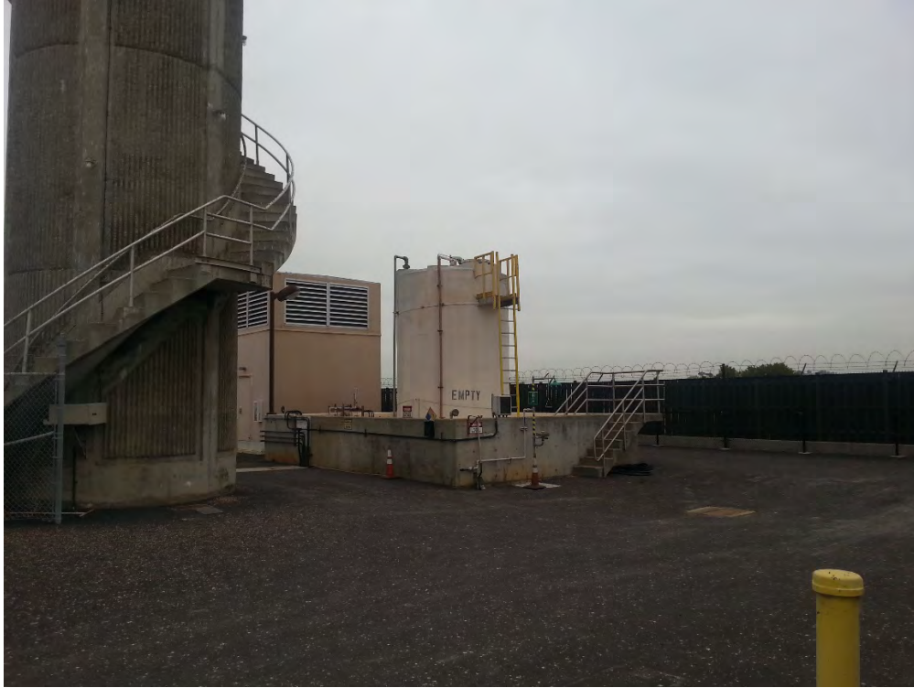
Figure 3 - Newark PS Chemical Storage Tank Located Within Containment Structure
