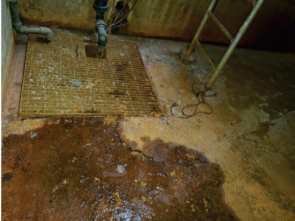
Figure 10 – Irvington PS Effluent Valve Vault: Damaged Area Around Sump
