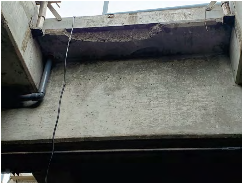
Figure 11 – Irvington PS Effluent Valve Vault: Spalled Concrete and Leaks at Access Hatch
