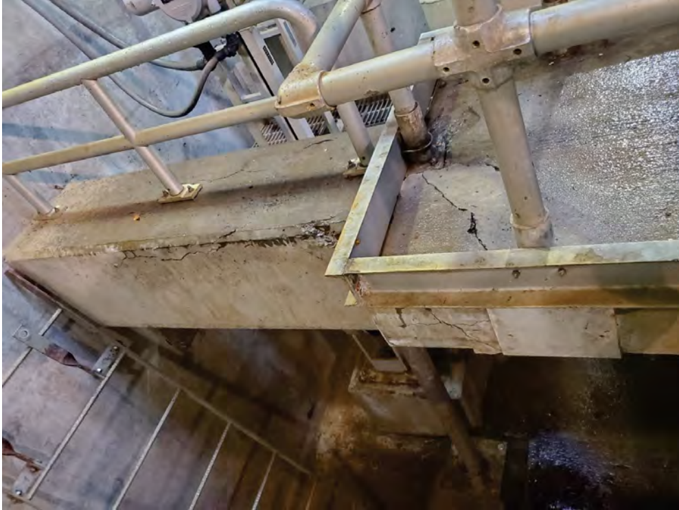
Figure 12 – Irvington PS Effluent Valve Vault: Spalled Concrete at Landing Platform Beam
