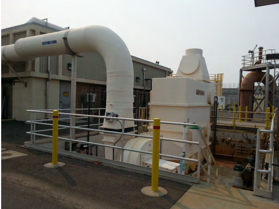
Figure 5 - Irvington PS Odor Scrubber Located Within Containment Structure
