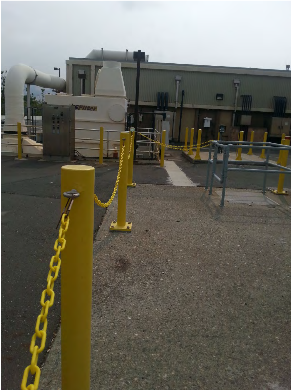
Figure 7 - Irvington PS Odor Scrubber (Background, Left) and Effluent Valve Vault (Foreground)
