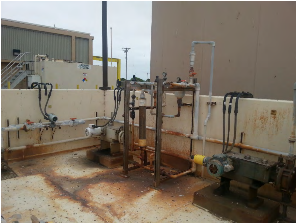
Figure 4 - Newark PS Chemical Metering Pumps and Distribution Piping Located Within Containment Structure
