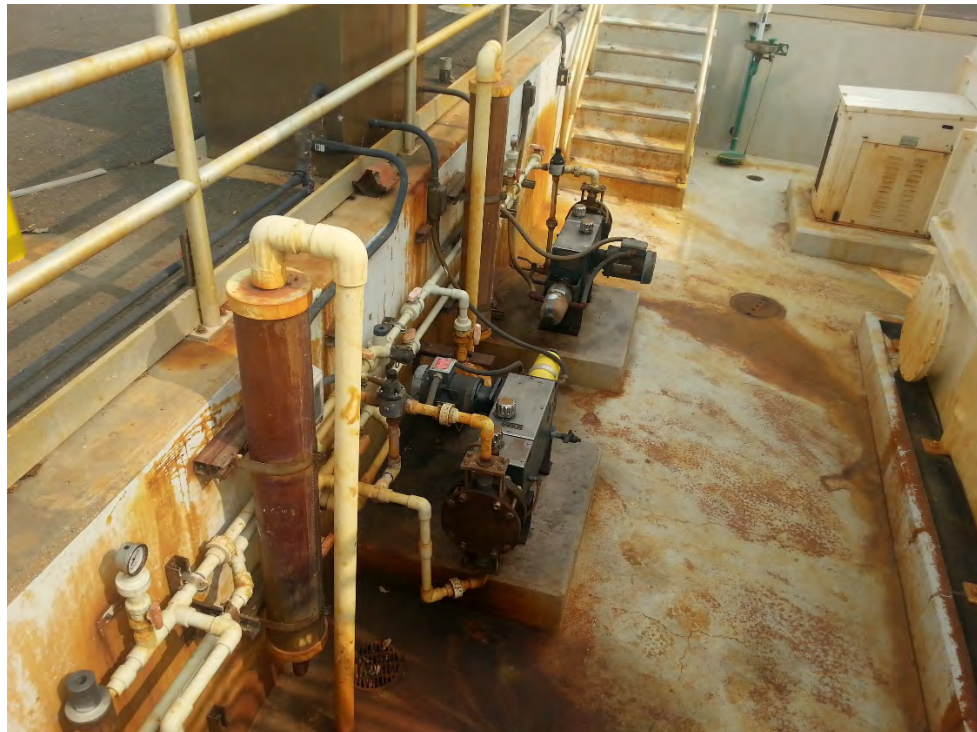
Figure 6 - Irvington PS Chemical Metering Pumps and Distribution Piping Located Within Containment Structure
