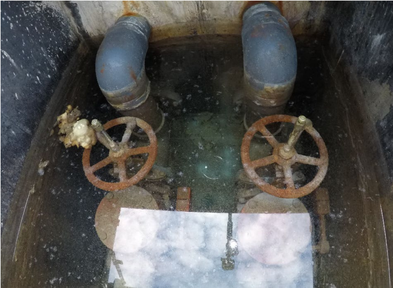
Figure 6 – Existing Valve Vault And Pump Discharge Valves
