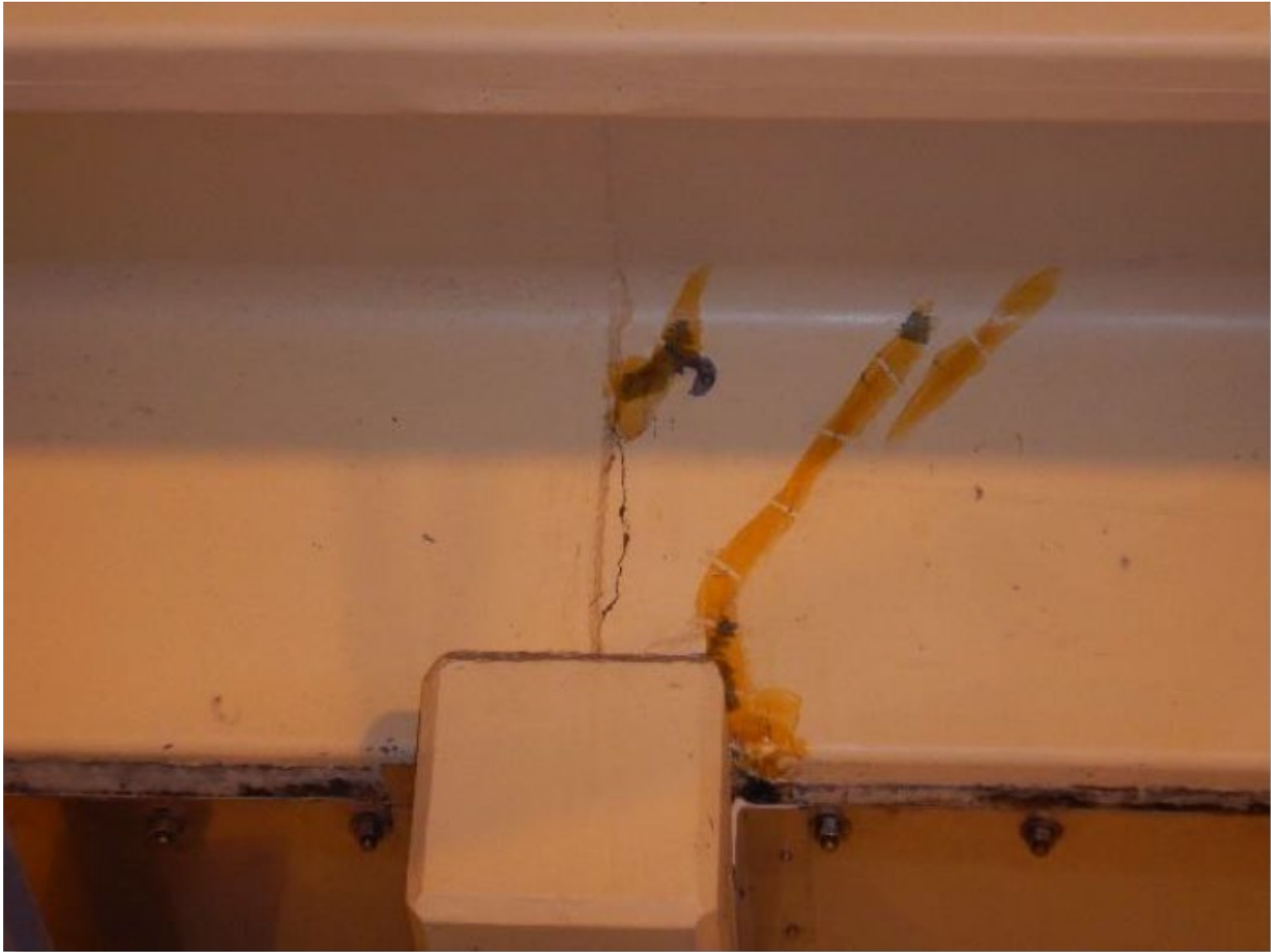
Figure 3 – Sludge Pump Room No. 1 – Cracked Roof T-beam
