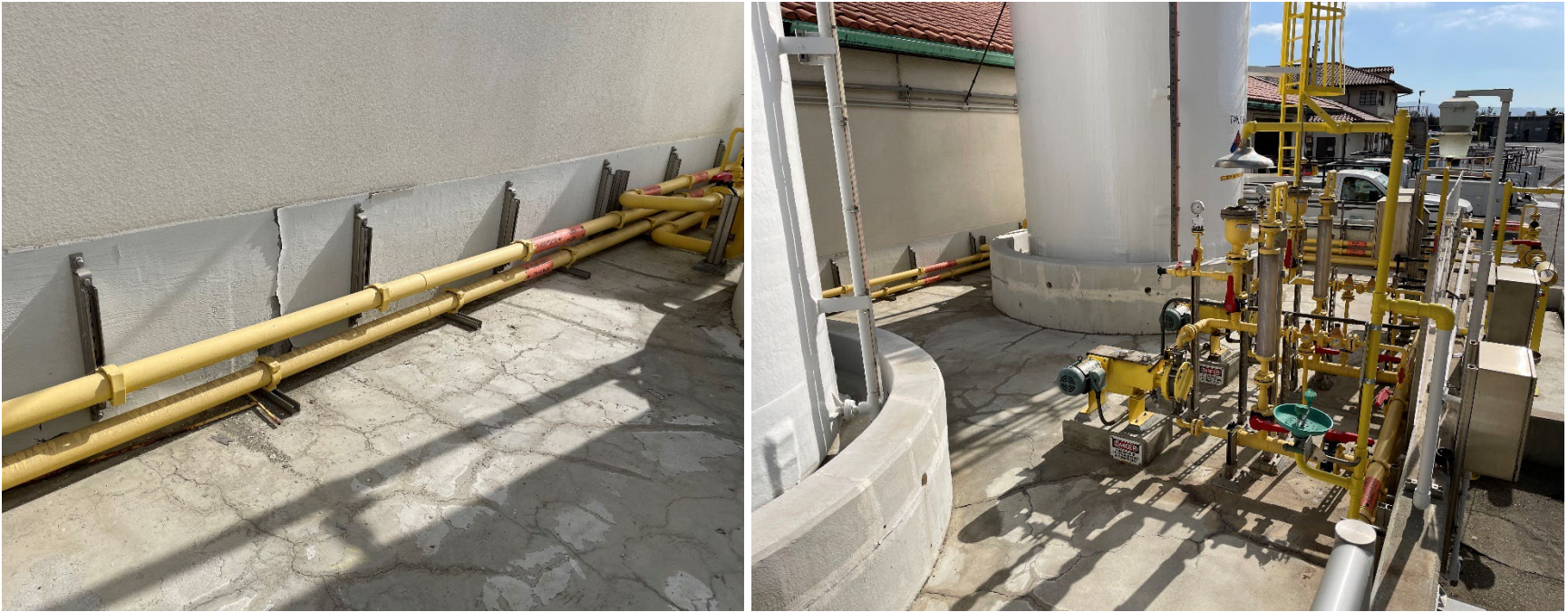
Figure 5 – Maintenance Shop Building Chemical Containment Area – Cracked and Delaminated Floors
