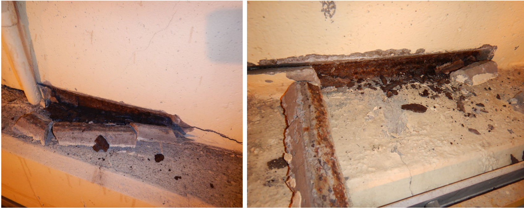
Figure 2 – Sludge Pump Room No. 1 – Spalled Concrete (Every three feet along wall)
